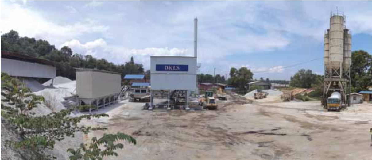
Premix Plant at Pundut, Perak
