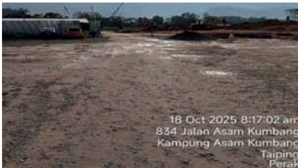
Provision of crusher run on access road to reduce dust and mud. Site roads are compacted evenly and regularly.
